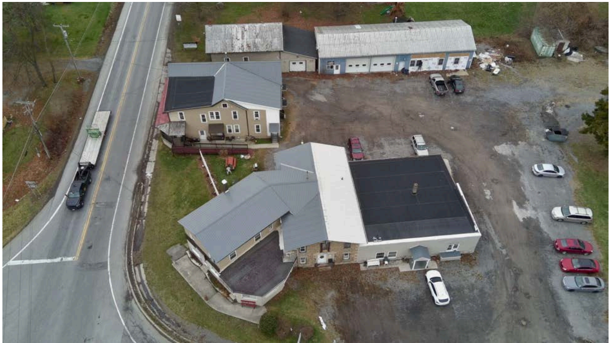
Photo F: View from corner of Route 63 and Route 36 along with a peak into current construction on the building. Windows, doors, new siding; the curb appeal will be significantly improved.
